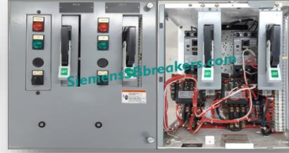
Siemens MCC Buckets
